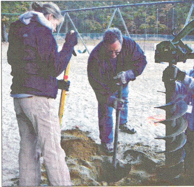
Rev. Ed Bove and Meghan O'Brien get to work finishing the work begun by an auger yesterday at Tiogue Elementary.
